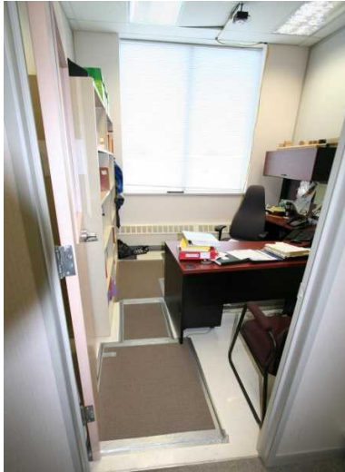
Figure 1. Example installation in office 19CN, showing temporary PIR sensor on the ceiling (black box), and pressure-sensitive floor mats (brown, edged with duct tape).
