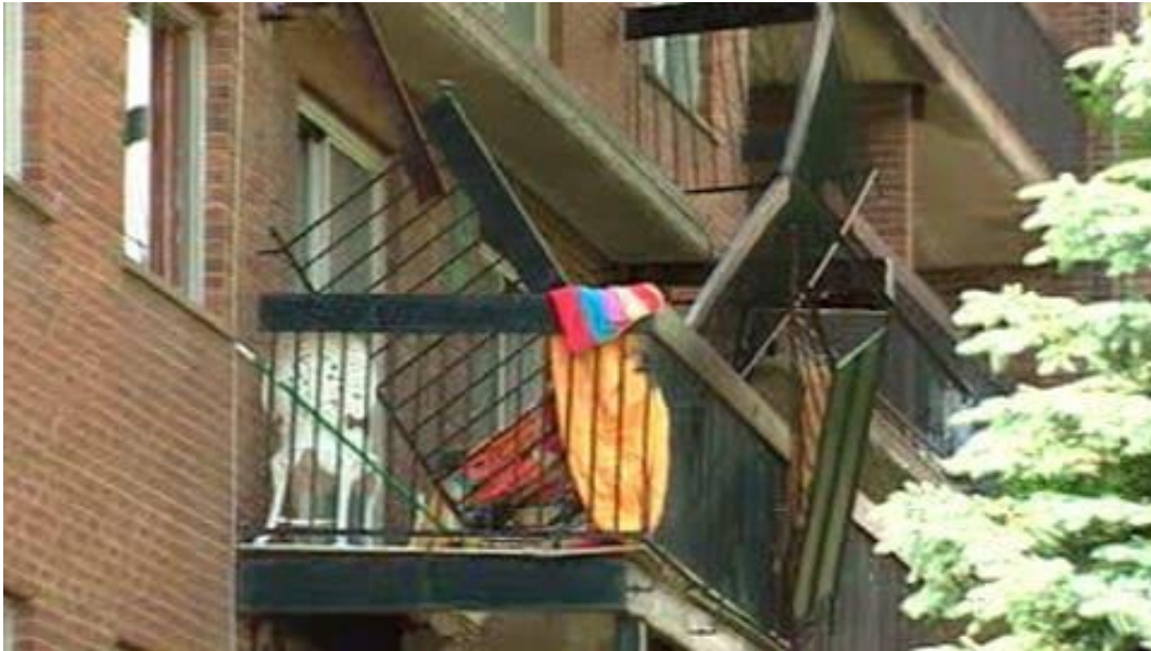
Figure 10: 2010 St-Laurent balcony collapse (Radio-Canada)
