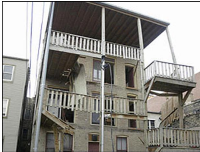
Figure 9: Chicago balcony collapse (AP)
