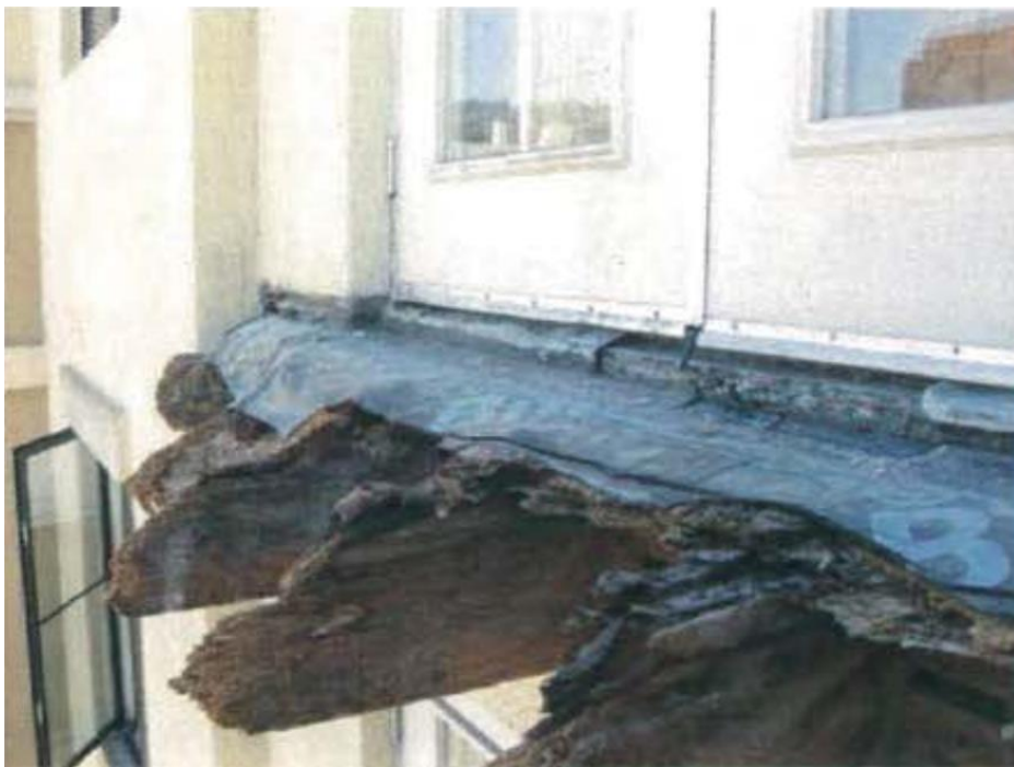
Figure 11: 2015 Berkley balcony collapse (CSLB)
