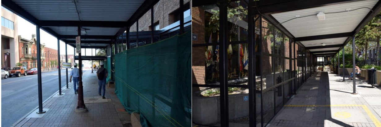
Figure 24 - Examples of pedestrian overhead protection located at the perimeter of TDLC.
