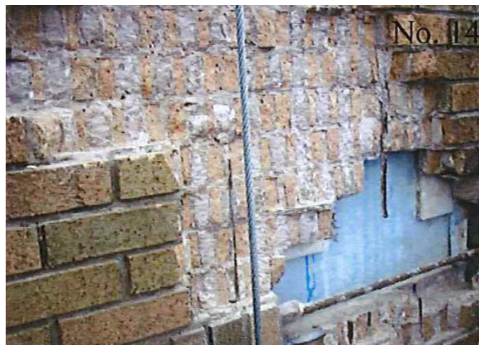
Figure 42 – Example of brick failure on wall panel
