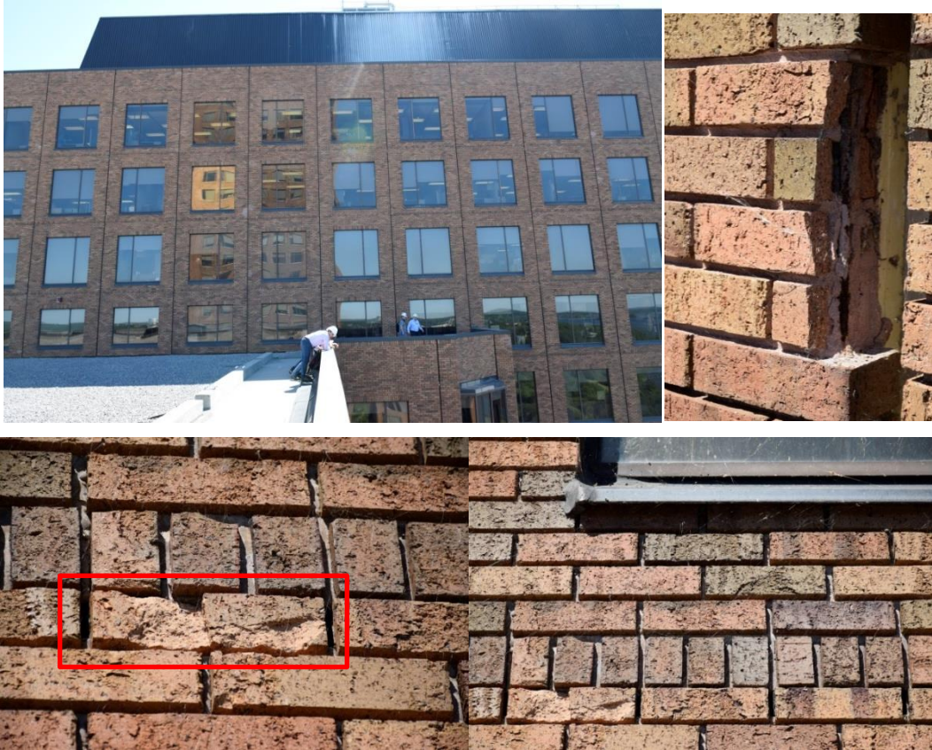
Figure 28 - Photos (Top-left) of elevation of West facing façade of Block 100 showing Roof (level 11) to Level 14; (Top-right) Evidence of brick fracture at panel joints; (Bottom photos) Details of brick spalling on East face of Block 100; Evidence of spalling of brick facia, likely due to freeze-thaw action; water run-off from window sill above wet portions of brick beneath sill making these locations more susceptible to freeze-thaw action
