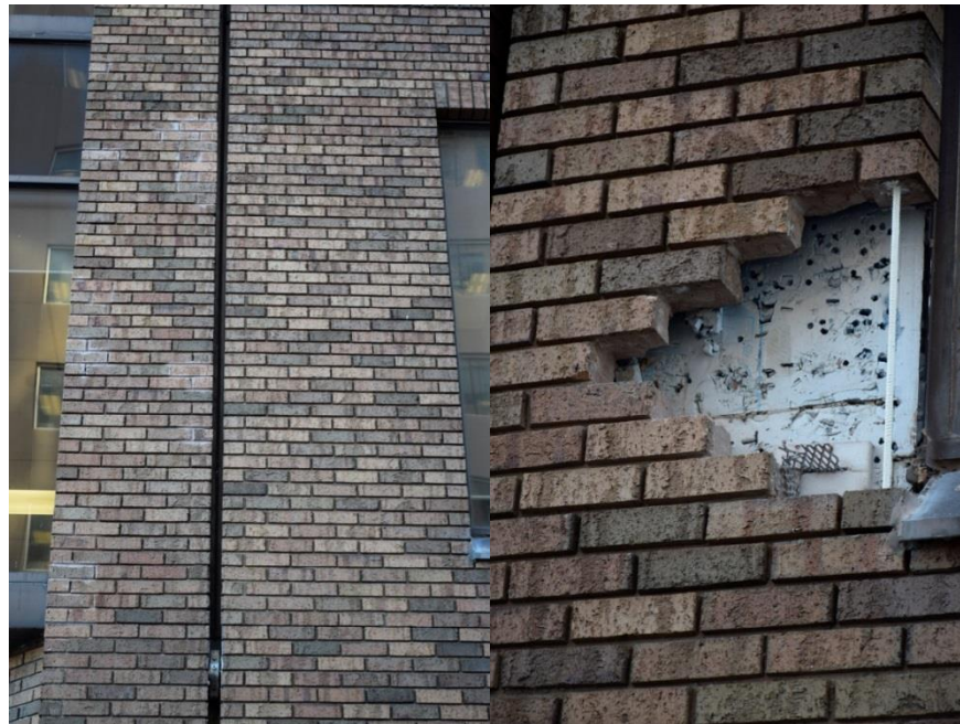
Figure 25 – Examples of repairs to brick units and brick veneer assembly conducted on East (Left) or to be completed on North (Right) façade of TDLC Block 100.
