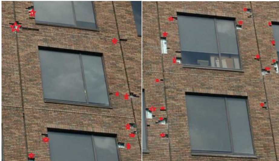
Figure 43 – Examples of brick damage at panel edges and window
