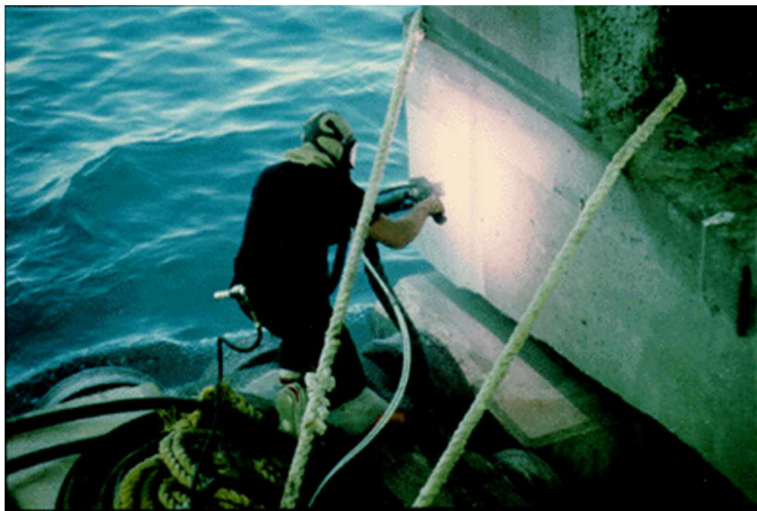
Figure 3. Arc spraying of zinc on a concrete bridge pier in the Florida Keys. In this case the zinc acts as sacrificial anode, although it is more frequently used in impressed-current systems. Three impressed-current zinc systems have already been installed by the Ministry of Transportation of Ontario in Toronto.
