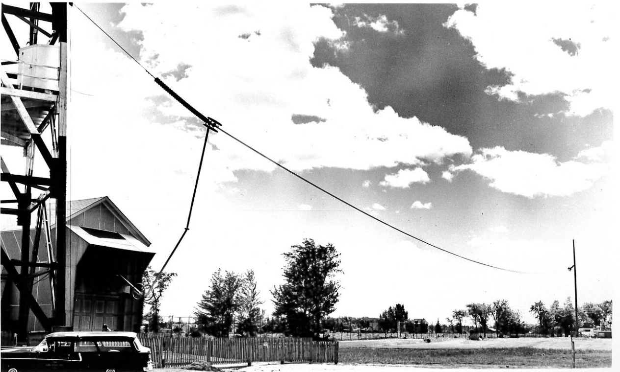
PLATE I — TEST LINE (above) single "Drake" conductor installed (below) two-conductor "Drake" bundle installed; spacing 18 inches
