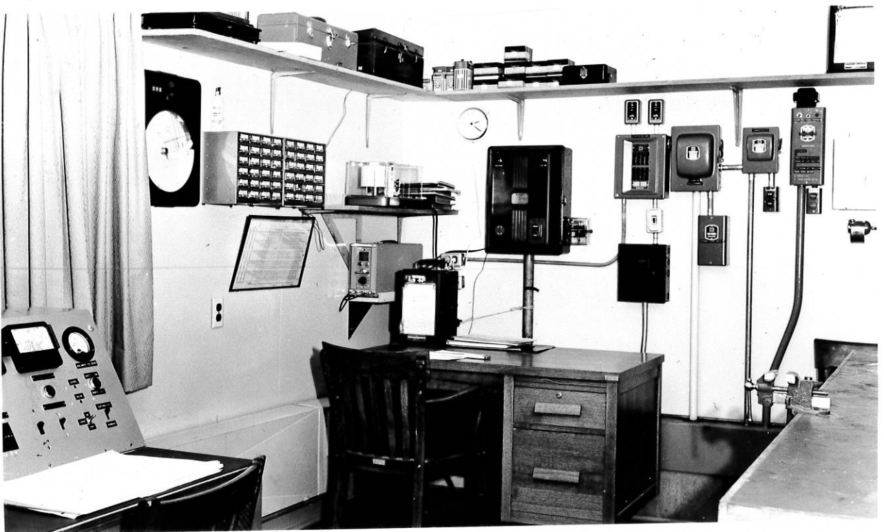
PLATE III — (above) High voltage supply and interior of high voltage building (below) Control room
