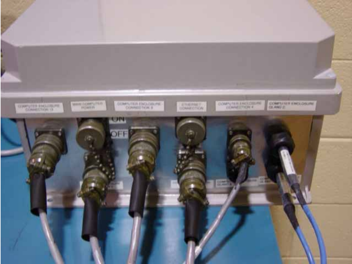
Figure 3. Computer Enclosure Exterior
