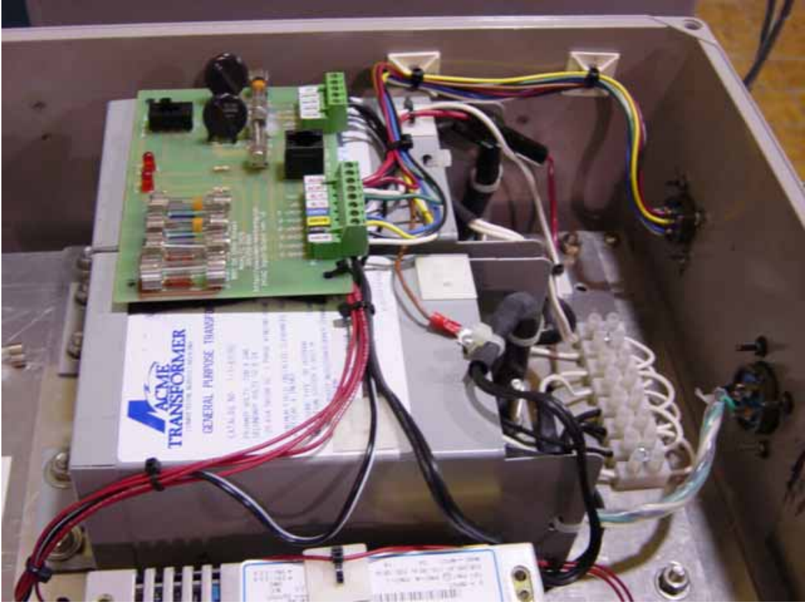
Figure 6. Power Enclosure Interior
