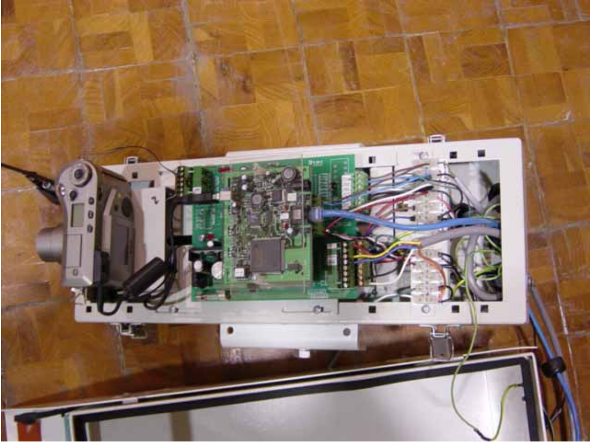
Figure. 10 Camera Enclosure Interior
