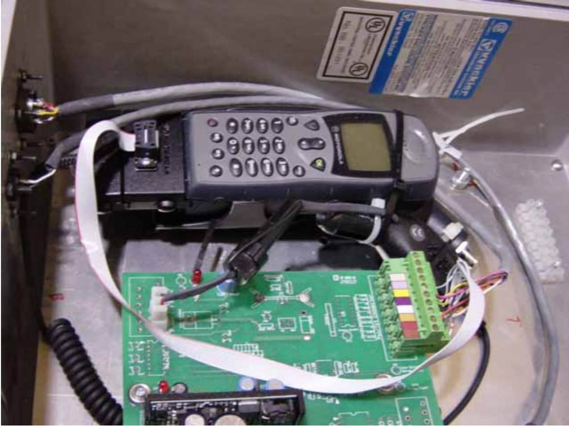
Figure 8. Telephone Enclosure Interior
