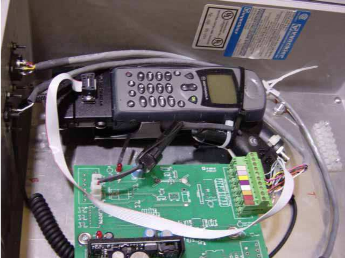
Figure 8. Telephone Enclosure Interior
