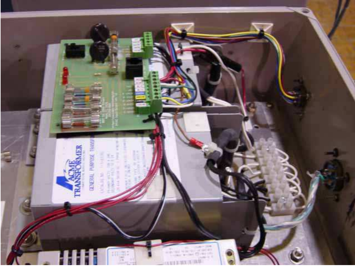
Figure 6. Power Enclosure Interior
