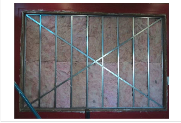
Figure 1. Reference wall assembly in test frame, with sheathing removed. The flat strap cross and bridging channel in the center of the wall brace against lateral and shear loads.
